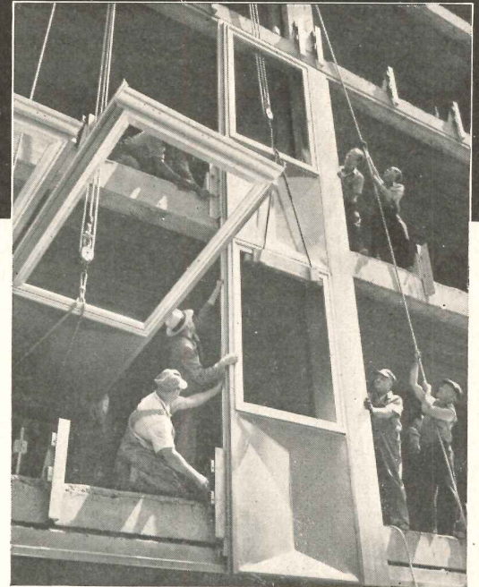
Workmen operating from inside of building, putting aluminum panel into position ready for bolting to steel brackets on framework.
