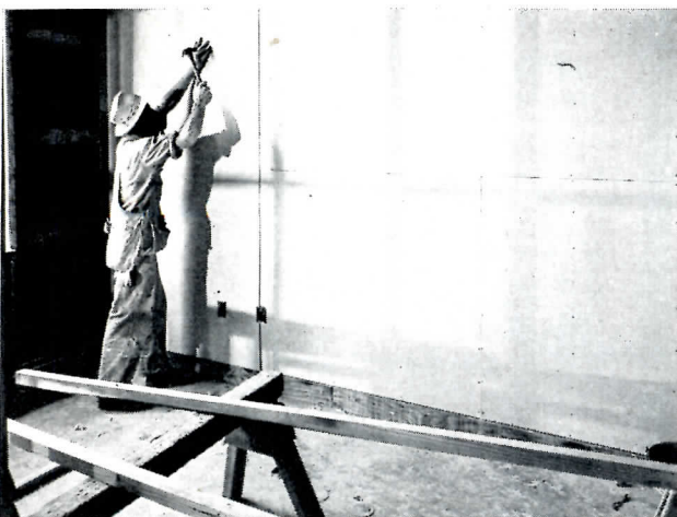
Temporary nailing of face layer. Minimum nailing holds panel until adhesive develops adequate bond
