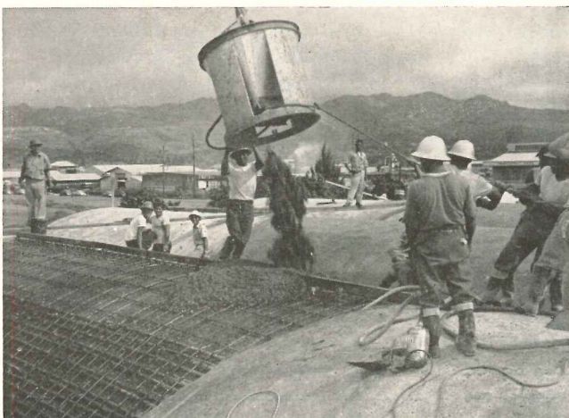
Here the middle and last section of a large barrel is being poured. The forms have screw jacks for raising and lowering
