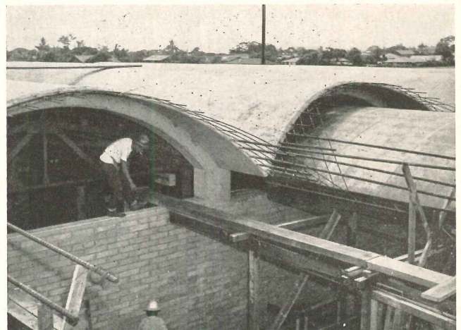
The form is being positioned for one of the three 32-ft barrels. Reinforcing steel projects to make a tie with the 93-ft shell
