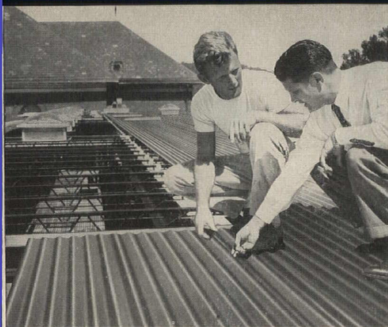
Deepest corrugation , \frac{3}{8} -inch, of all standard steel centering is available with Fab-Form. Job Superintendent Thomas A. Laboon, left, shown with Pittsburgh Steel Products Salesman C. W. Bainbridge Jr., said deep corrugation helped make a stronger slab.
