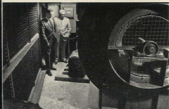
Fan room equipped with series 8000 Air-Foil centrifugal fan and air conditioning coils. W. Y. Humphreys, Westinghouse, with John Mullin, Consulting Engineer, air conditioning and ventilation system designer.
