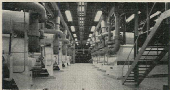
Rows of white absorption chillers with their color-coded piping taking their reactivating energy from high temperature water
