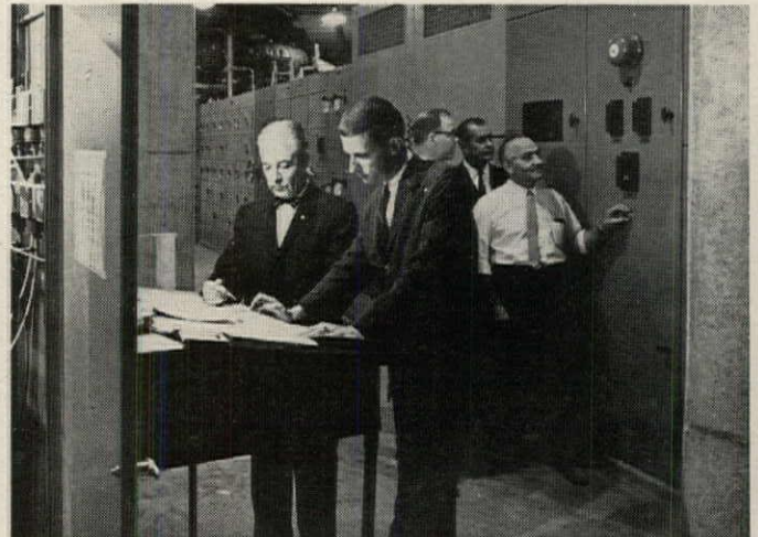
Checking construction progress are C. J. Long and F. J. Sarknas, Westinghouse. In background, 1500 kva power center supplies power for building auxiliary and air conditioning compressor motors.
