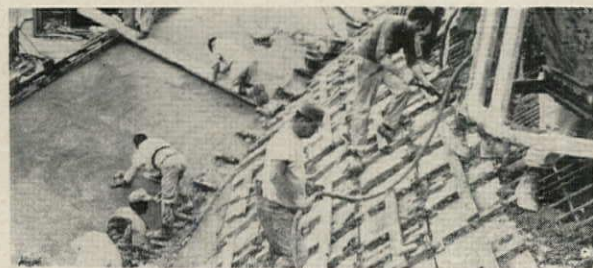
Leap-frogging counterforms creep up steep TWA sides as pourers lead and finishers follow, a timing tour de force to make a monolithic shell in one pour
