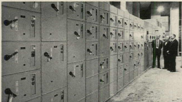
Westinghouse Motor Control Center located in the Mechanical Room centralizes auxiliary motor controls. Discussing installation advantages are H. R. Helvenston, C. J. Long and N. J. Grady.
