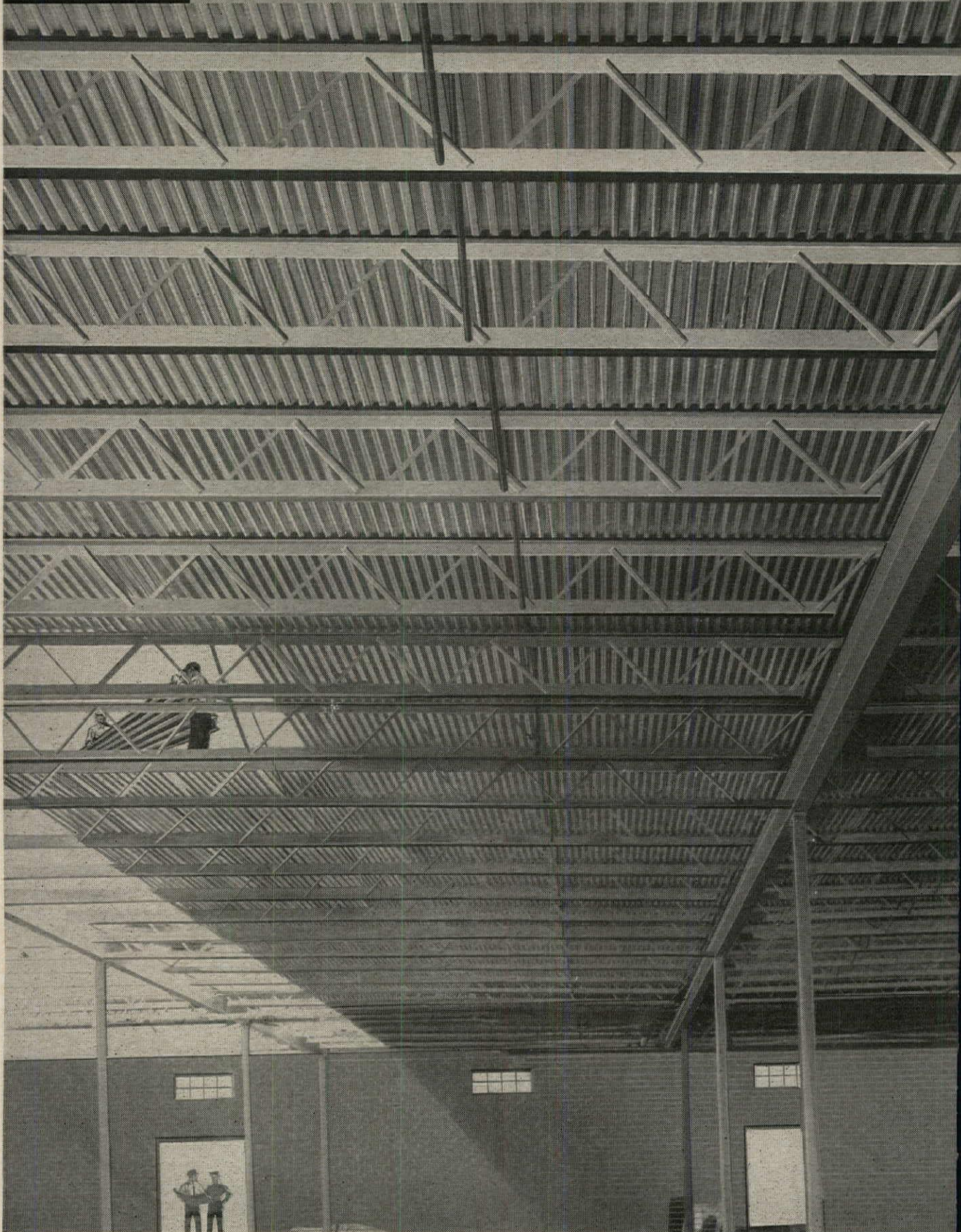
Tensilform complies fully with American Iron and Steel Institute's Design Manual for Light Gauge Structural Shapes (1960 Edition).
