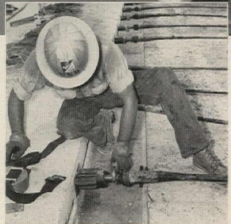
Use of coupled tendons allowed reduction of pour size, minimizing shrinkage and creep losses.
