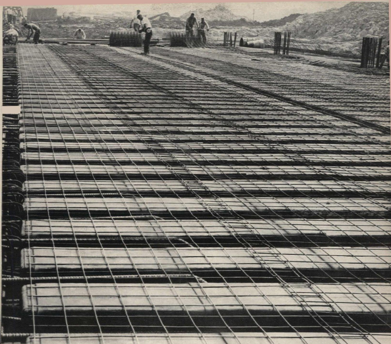
Typical forming for monolithic Ceco concrete joist and beam construction is seen in this construction view of the Terminal Building at O'Hare International Airport, Chicago. These are Flangeforms, ready for concrete pour.
