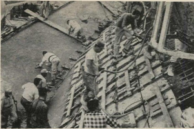
A water-reducing, retarding admixture was used in concrete at Eero Saarinen's T.W.A. terminal at Idlewild to permit finishing upon removal of counterforms, while the mass of the
