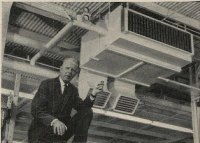
COMBINATION ELECTRIC UNITS suspended from roof provide air conditioning in summer and have built-in resistance coils for winter heat. Chief Engineer Russell Bush points out their compactness.
