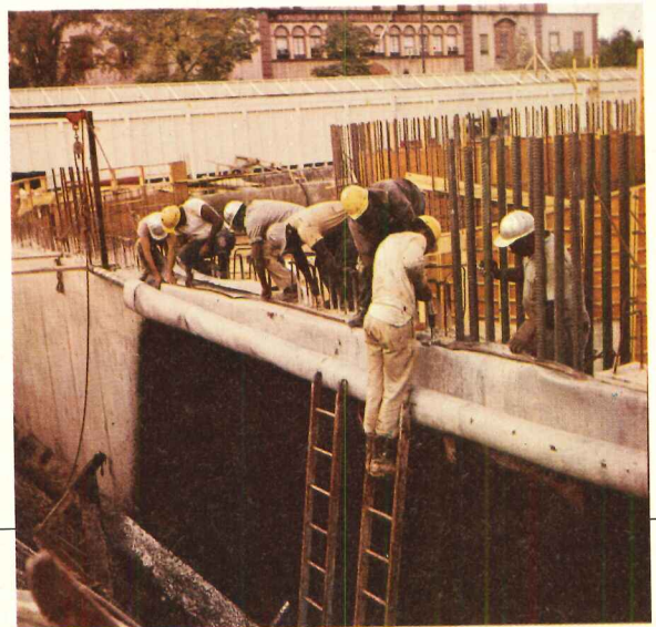
Workmen installing 20' x 90' Butyl sheets to form watertight sack before foundation was poured. Butyl sheeting material manufactured by Carlisle Corporation, Carlisle, Pennsylvania.
