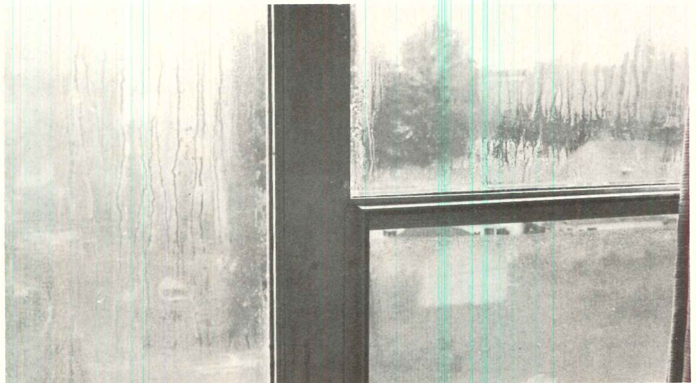
Condensed moisture within the air space—a sure sign that the insulating glass seals have failed.
