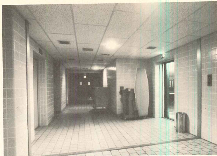
Service corridor during emergency has one freight elevator operating plus center row of incandescent fixtures and all exit and stairwell signs.
