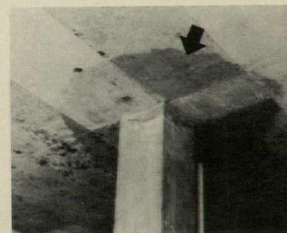
Detail shows contrast between 9000 psi column concrete (in the slab immediately adjacent to the column) and 4000 psi flat-plate floor concrete.
