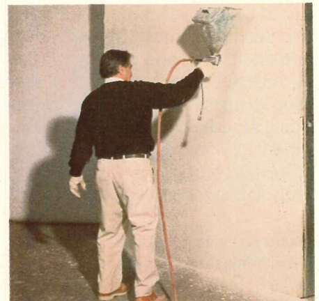
attractive, textured finish coat is sprayed over the prime coat. Both prime and finish coats can be troweled or sprayed. The result is superior insulation and the attractive finish shown at the right.
