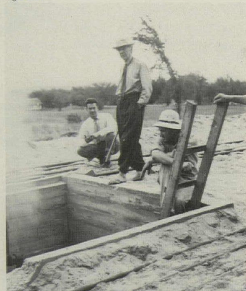
Frank Lloyd Wright inspecting the floor heating pipes in the Jacobs House, Madison, Wisconsin.
