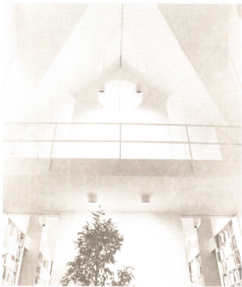
Ceiling ridge with open seam
