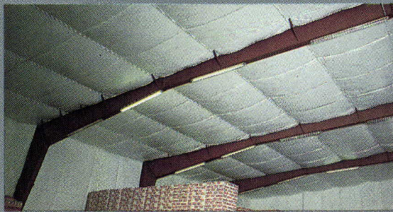
The Energy Miser system at work—St. Petersburg Beverage Company, Largo, Florida.
