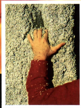
Mineral Wool Sprayed Fiber
