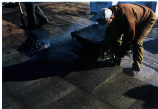
A Tapered FOAMGLAS® Roof Insulation System was specified for the re-roofing of the library.
