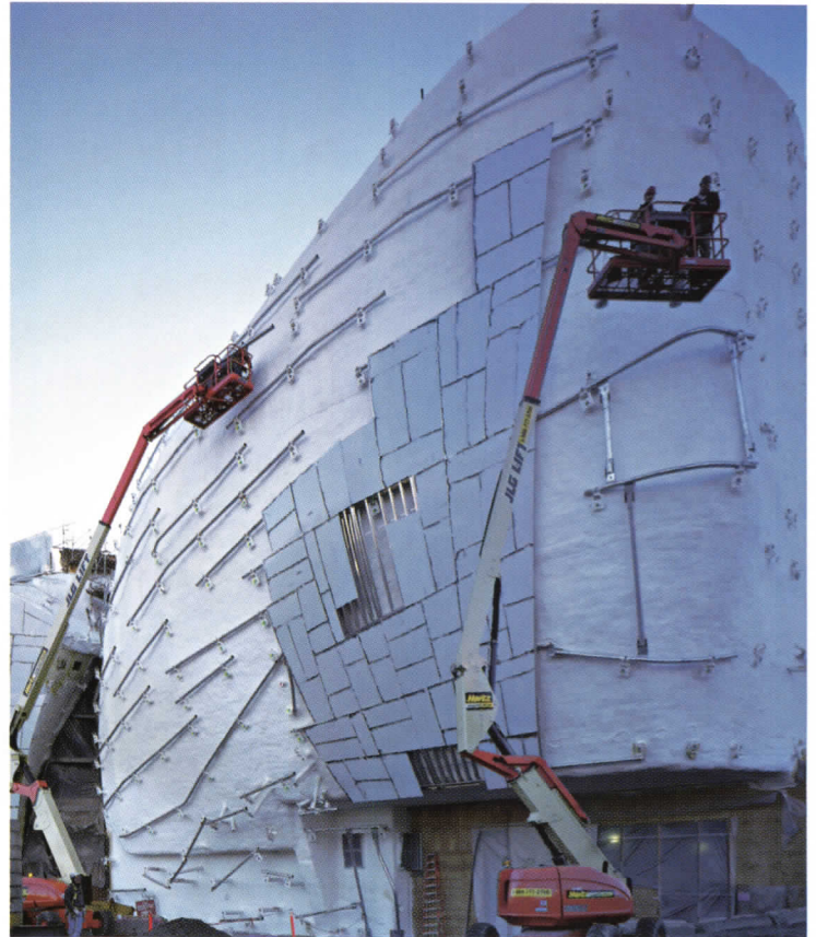
Five-inch aluminum pipe girts, which could be adjusted four inches in any direction at either end as required to locate them precisely, were first anchored to structural pedestals. Next, the metal panels were installed.
