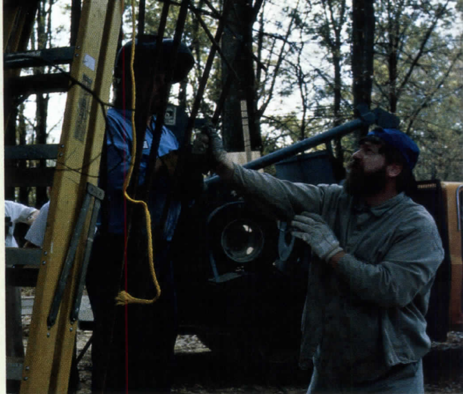
Sambo working on the tractor shed, Flautt House, Greenwood, Miss., Mockbee Coker Howorth Architects, 1988.
