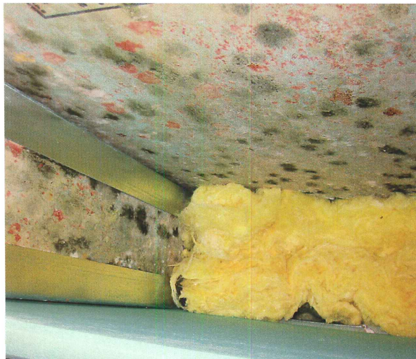
A wall cavity in a building under construction in the Northeast developed mold because materials were not kept dry prior to installation and water was entering from upper stories as they were being built.
