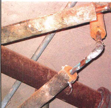
Moisture control is the key step in halting mold growth in buildings (171).
