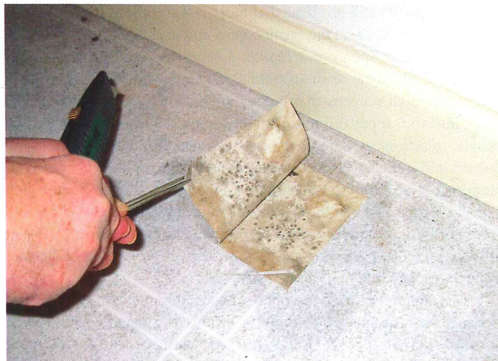
Mold grows under sheet vinyl covering a concrete floor in the Midwest because a vapor barrier had not been placed below the slab during construction, thus allowing ground moisture to penetrate the concrete.
