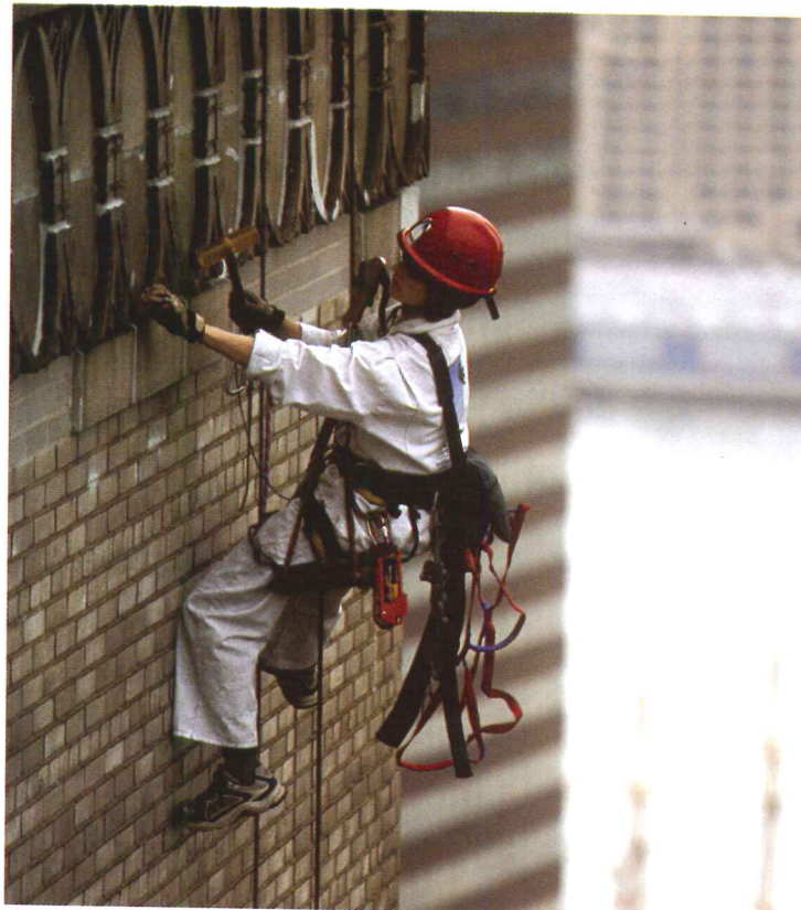
A surveyor, suspended by a two-rope system similar to that used by climbers, evaluates and documents facade conditions of a historic building.
