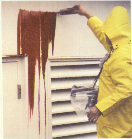
The owner of a former warehouse found evidence of water penetration in the building's mechanical space (left middle and bottom). Water testing (left) ruled out leaks in
