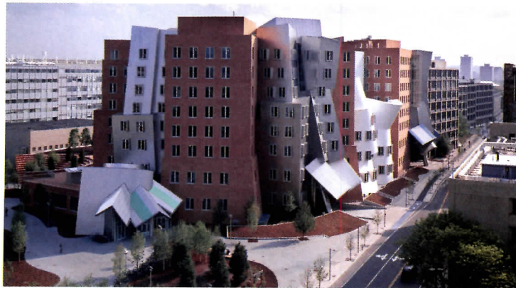
MIT's suit alleges that the Stata Center has developed "persistent leaks," and that ice and snow slide from the roof during winter and present a hazard.
