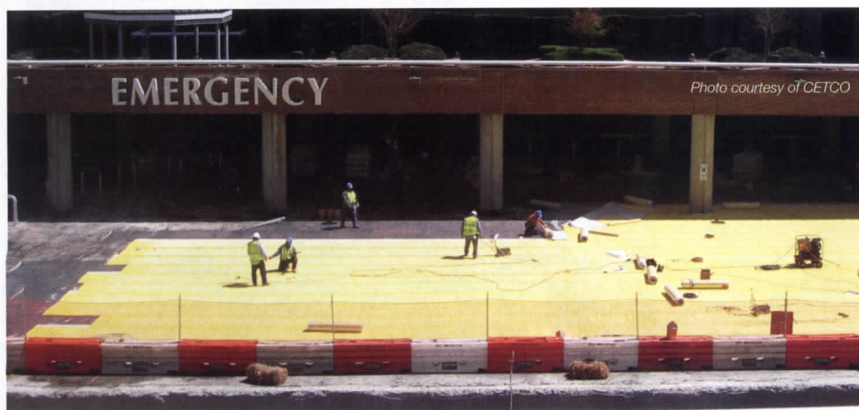
Workers installing thermoplastic membrane waterproofing system over the existing failed rubberized asphalt membrane on the split-slab deck of this hospital.
