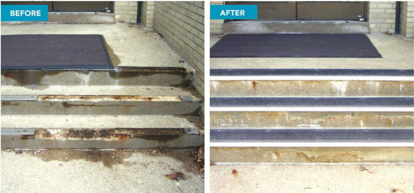
Left: Concrete stairs show their deteriorated condition before using renovation treads. Right: The stairs—with new renovation treads installed—have been restored to a safe condition.
