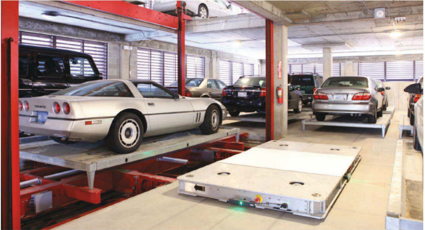
Robots store and retrieve cars on steel trays in this latest-generation automated parking system in Crystal Springs Resort, Hardyston, New Jersey.
