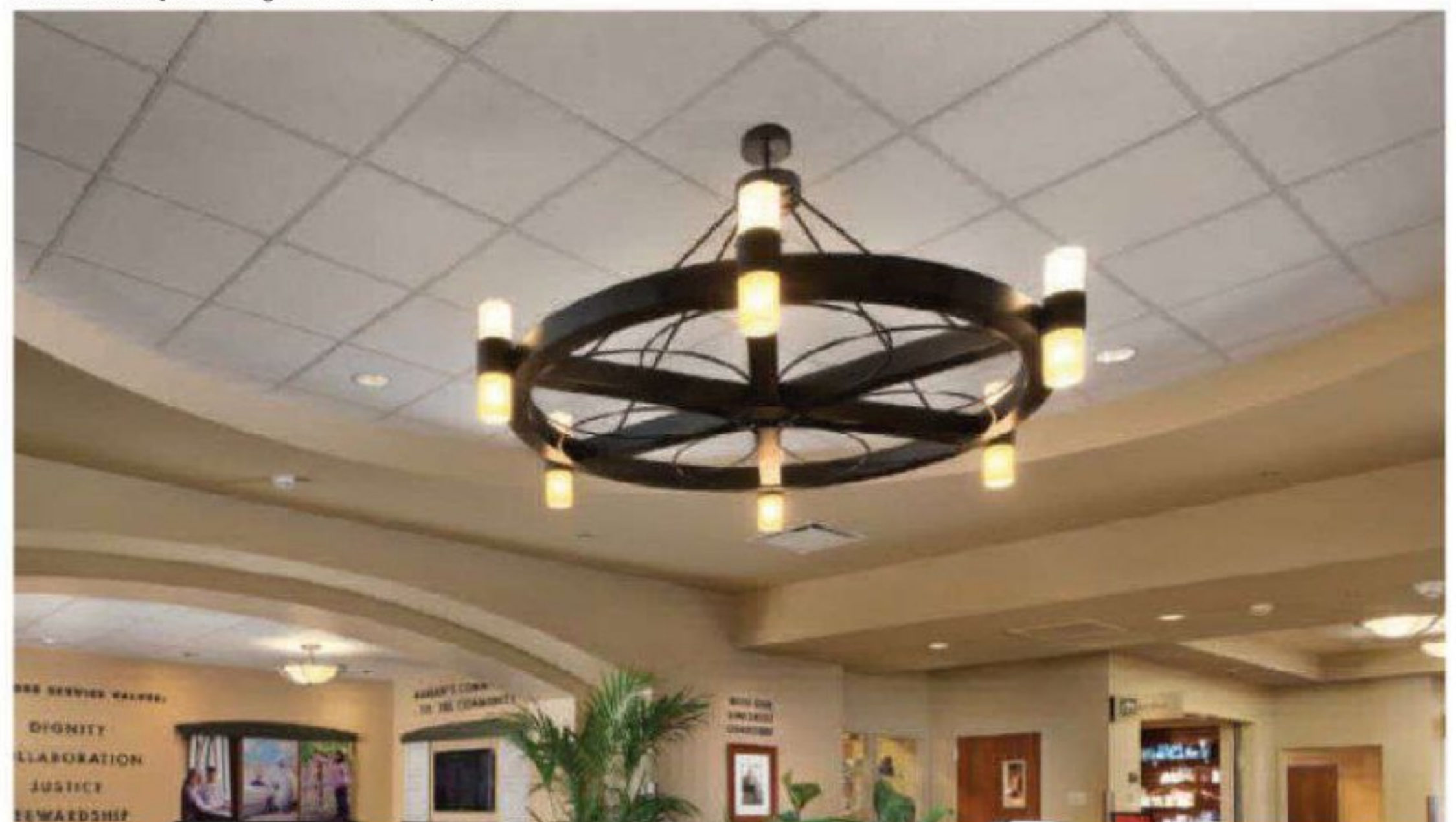
At Marian Regional Hospital in Santa Maria, California, seismic performance was a factor in Moon Mayoras Architects’ choice of a suspended ceiling system.
