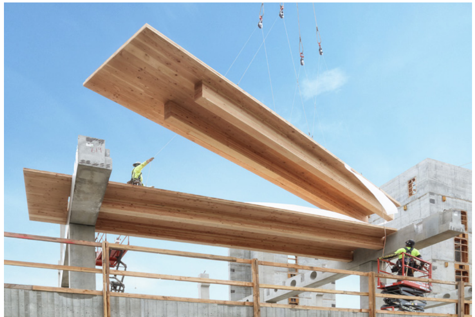
FIGURE 5 – Adidas North American HQ utilized a pre-cast concrete frame with prefabricated mass timber floor decks to reduce construction costs and schedule for a financially viable project. Image: LEVER Architecture
