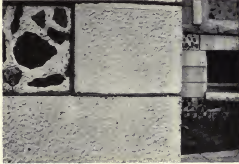
An Excellent and a Poor Example of Concrete Finish. The Corner Stones Are Finished With the Pointer and Appear Well. The other Stones Have Aggregate of Too Large Size Impressed Into Surface.
