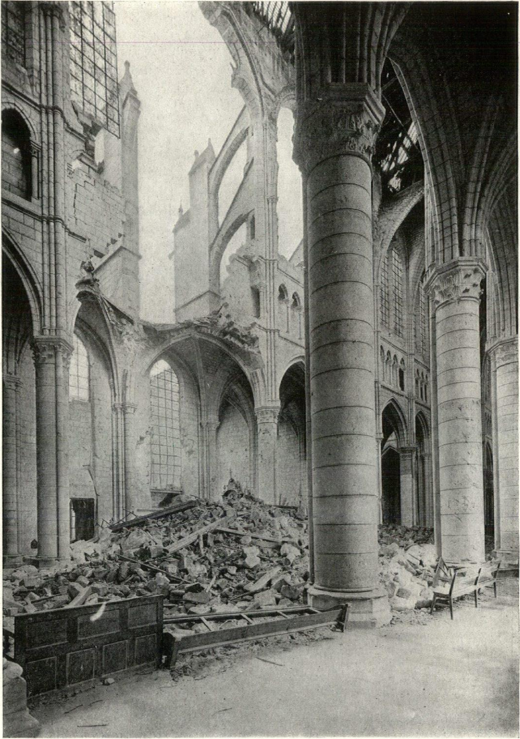
THE RUINED BAYS FROM THE SOUTH AISLE—SOISSONS CATHEDRAL.
