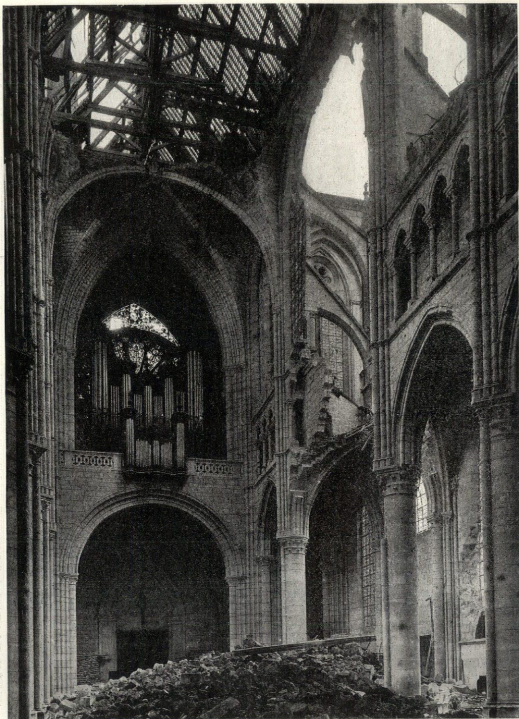
VIEW LOOKING NORTHWEST, SHOWING DESTRUCTION OF CLEARSTORY AND TRIFORIUM OF SECOND AND THIRD BAYS—SOISSONS CATHEDRAL.
