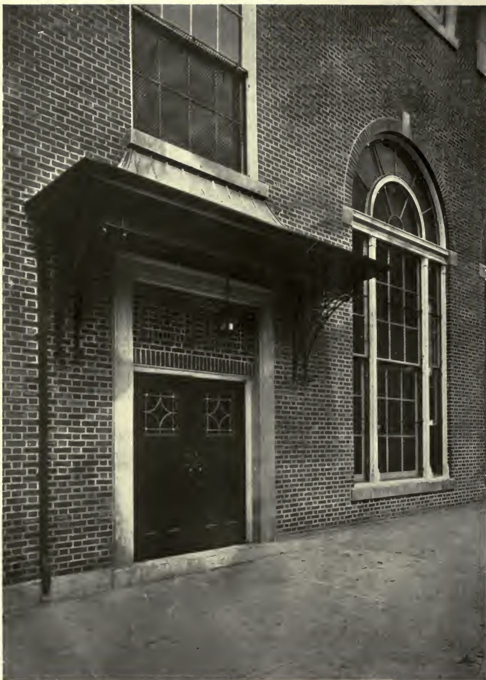
DETAIL OF SIDE ENTRANCE—THE NEW LINCOLN HIGH SCHOOL, NEW YORK CITY. STARRETT & VAN VLECK, ARCHITECTS.
