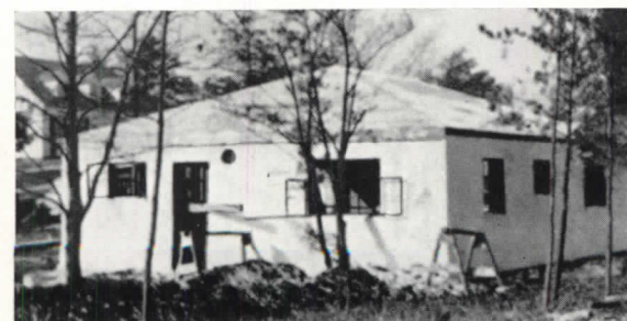
Finished structure is monolithic, with finish bonded to a wall consisting of two 3" elements with 5" air space between. For details of vacuum process, see March 1936, page 239; September 1936, 242.
