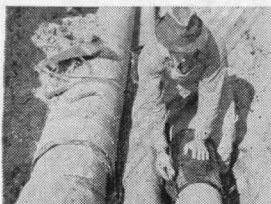
Installing connector band. All necessary accessories are pre-fabricated and shipped with order.
