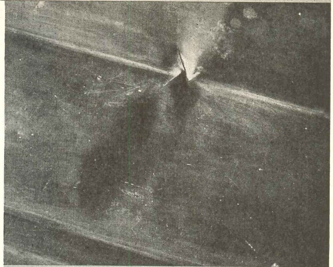
The same gutter after 12 cycles of heating and cooling. The pinch has now developed a visible crack in the copper. The temperature range for each cycle exceeded Nature's 150° change from maximum in summer to sub-zero in winter, and it is thus estimated that each cycle in the laboratory is equivalent to one year of actual service.
