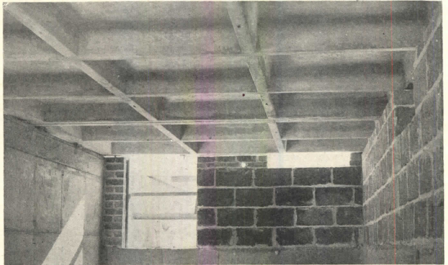
Basement view of precast floor slabs. The slabs on upper floors are also left as exposed ceilings, after painting. Joints are pointed and marginal ribs set flush with walls
