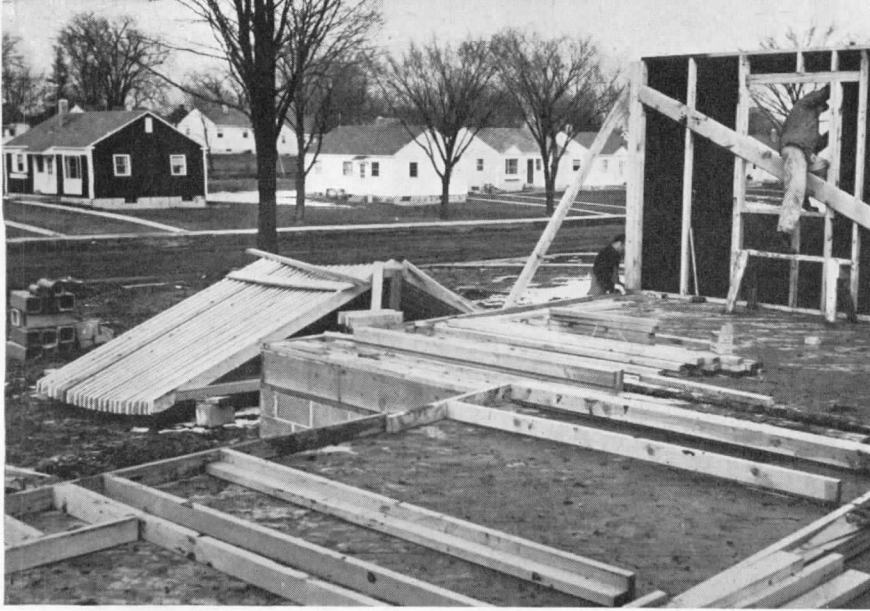
Above: walls being assembled on subfloor, one wall in place, roof trusses in background
