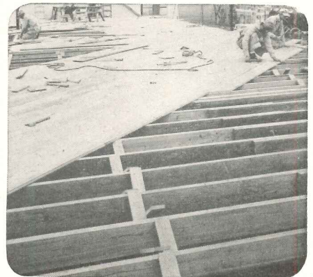
3. Wood used in or near the ground open to attack by termites.
