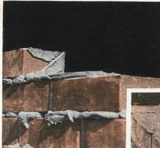
Nail holes frequently connect with voids in the head joints which in turn connect with unfilled furrows in the bed joint.
