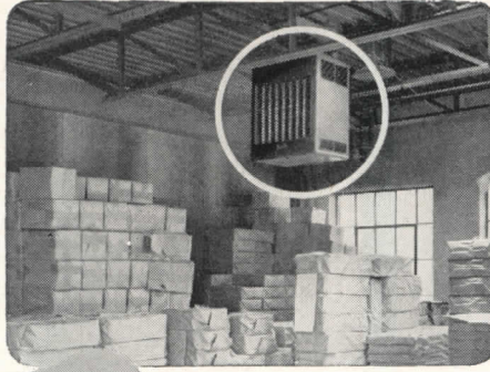
This stockroom added to original building couldn't be heated from main plant. A single Janitrol unit answered the problem.
