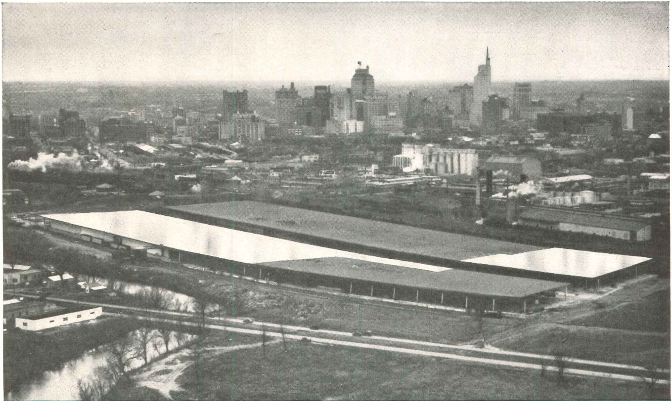
ALFORD REFRIGERATING WAREHOUSES, DALLAS, TEXAS — NOW UNDER CONSTRUCTION, ROOFING CONTRACTOR: LLOYD GRAY, MT. AUBURN ROOFING COMPANY. SPECIFICATIONS FOR THE 23 ACRES OF BUILT-UP ROOF: 2 PLYS OF REYNOLDS .004" EMBOSSED ALUMINUM OVER 30 LB. FELT
