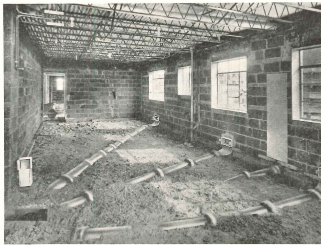
In basement suites, return air is brought back to furnace through return grilles under windows which lead into vitreous clay pipe
