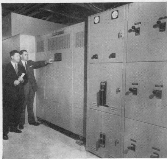
FLEXIBLE double-ended load center unit substation with integrated units furnishes highly dependable power close to load.
