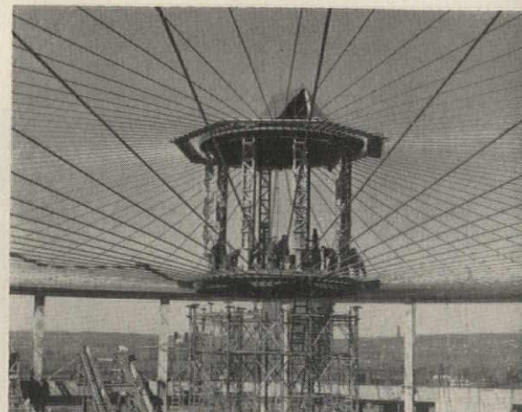
Right: rings are about at their final position and are ready for 5-in. pipe spreaders to be inserted. Detail above indicates how this was done
