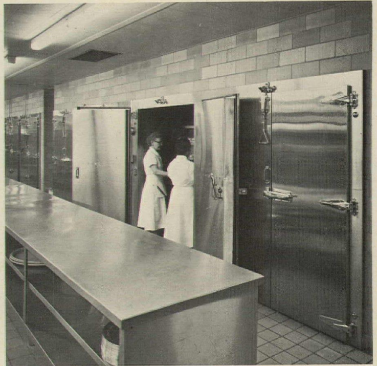
Jamison FS double cooler and freezer doors in hotel kitchen are completely stainless clad for easy cleaning and bright appearance.
