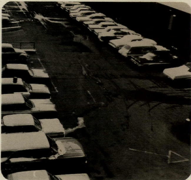
PARKING AREA BEFORE AND AFTER a Revere Snow Melting System has been installed. Imagine the mess here, trying to plow out so that cars can park. Photo with tube exposed shows grid-type installation.
