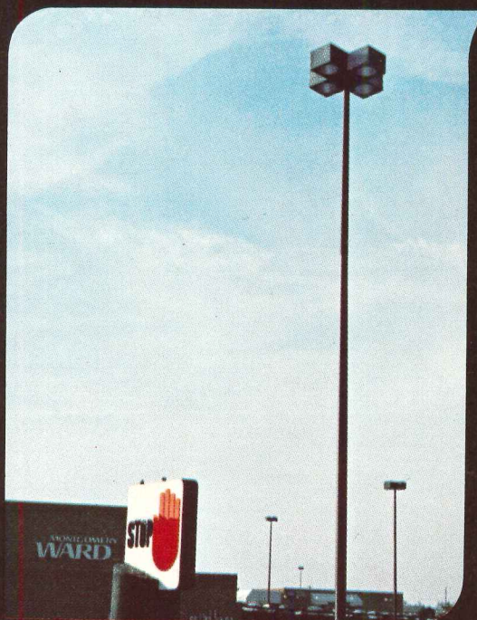
For large areas, SCL series luminaires keep the light on the ground, not in your neighbor's eyes. Its high efficiency gets the most light to the need, economically.
