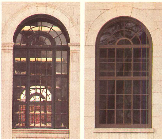
Required costly maintenance; old windows inefficient. Wide muntins cut visibility.
