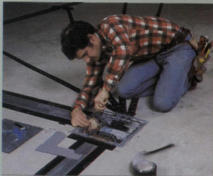
New AMP floor distribution box.
