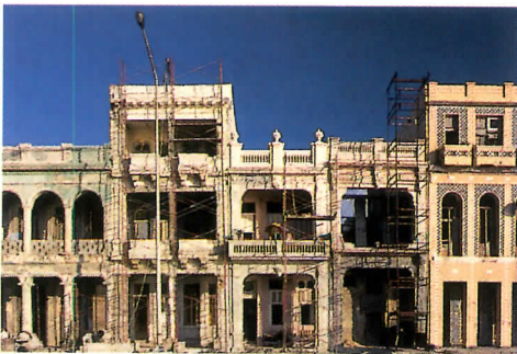
Portions of Malecón, the waterfront jetty of Old Havana, undergoing restoration (above and right).
