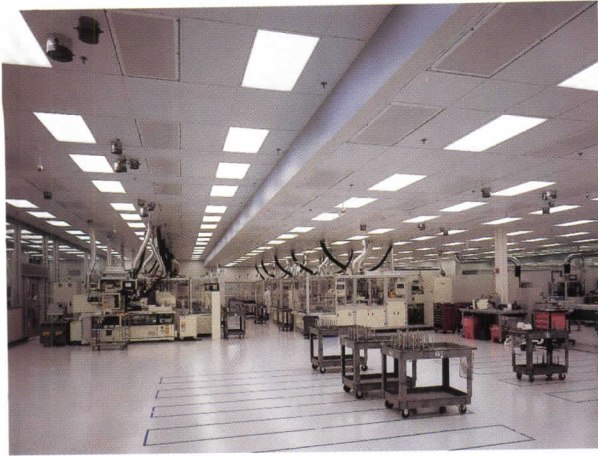
Printing and replication areas (above) needed lighting that met clean-room standards and gave uniform illumination over floor areas. The staging area (right)
