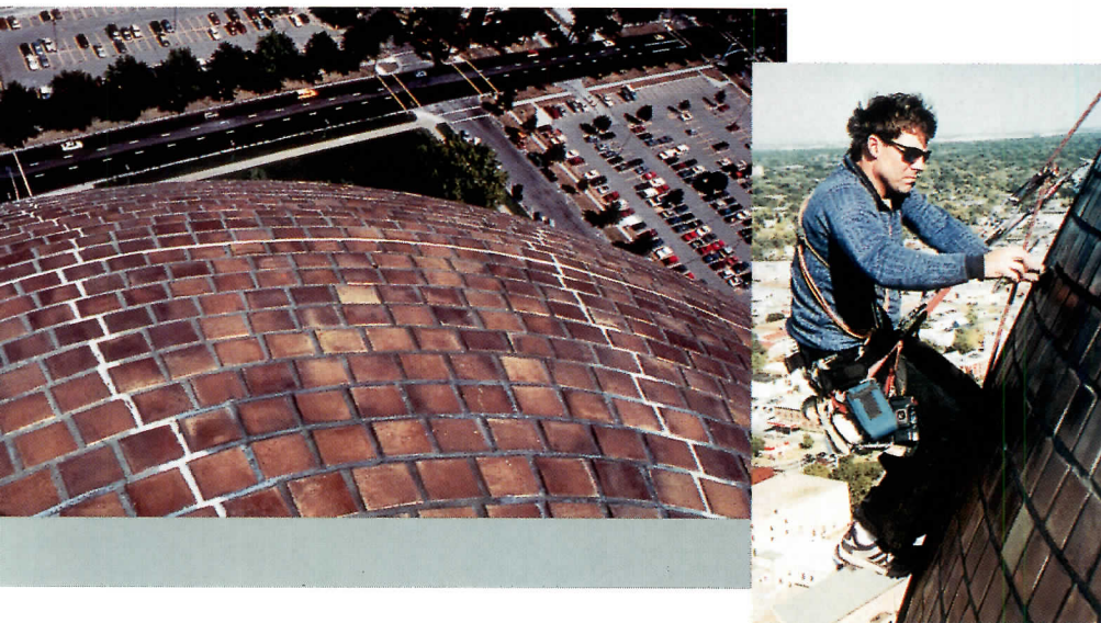
RAPPELLING FROM THE SOWER, A STATUE atop the capitol dome (left), field inspectors performed visual inspections and applied nondestructive testing methods to examine cracks in the dome (far left) and assess the tower's condition.
