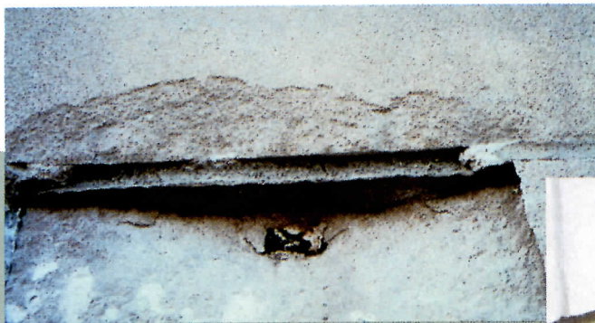
THE STONE IS SPALLED AT SOME JOINTS where ties bind the expanding masonry to the shrinking steel frame (above). Test panels were cleaned using nondestructive methods (right).
