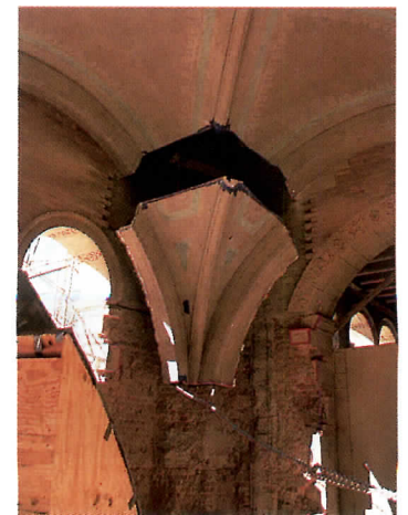
Removing the corners of the vaulted ceilings beneath the towers provided access to supporting piers.
