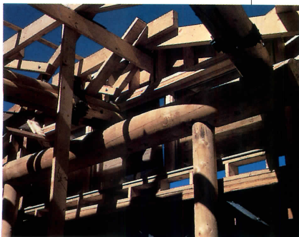
RoTo’s student center integrated prefabricated building modules (above left), stripped to their steel frames. Straw bales (above right and opposite left) became an infill wall, built by local junior high students. During construction, other tribal members honed such skills as timber framing and carpentry (this page, bottom).
