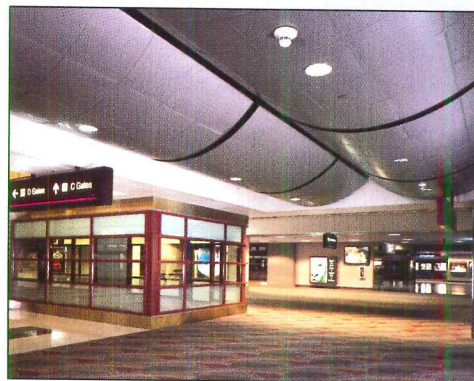
The CURVATURA 3-D Ceiling System from USG adds drama and visual interest to the McCarran International Airport, Las Vegas, Nev.
