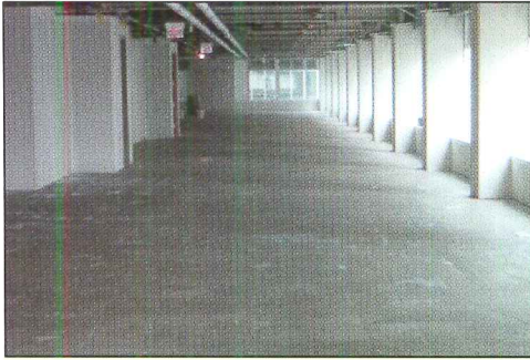
The existing concrete floors in this renovated 26-story office building in downtown Philadelphia were cracked and uneven.
