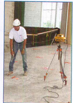
Barrier Corp. flooring applicator crews used a laser to measure existing floor elevations.
